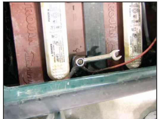
22. Positive Battery Connection
